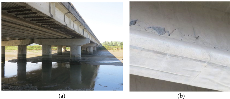
Figure 1. Photograph of the investigated bridge: (a) side view; (b) cracks along the tendon duct.
