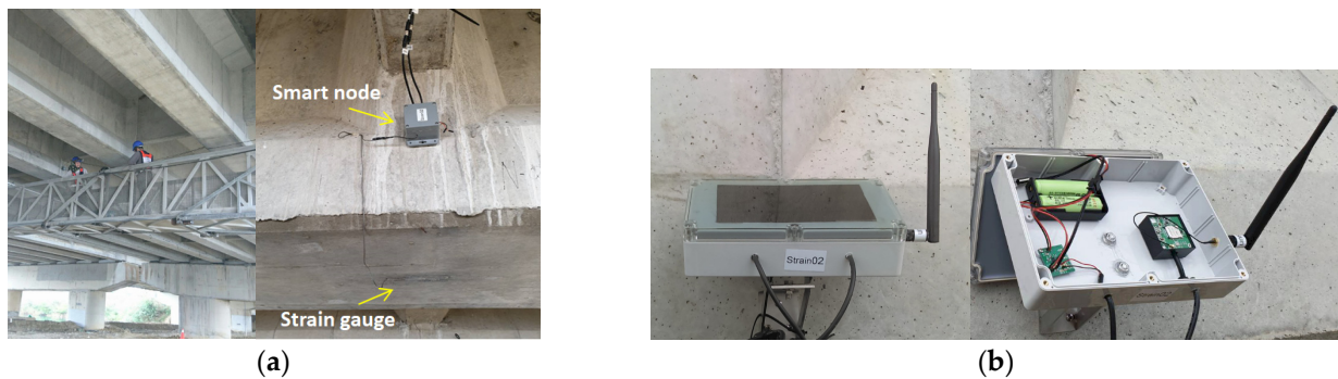
Figure 15. Dynamic strain monitoring device: (a) on-site installation; (b) solar charging panels with rechargeable batteries.
